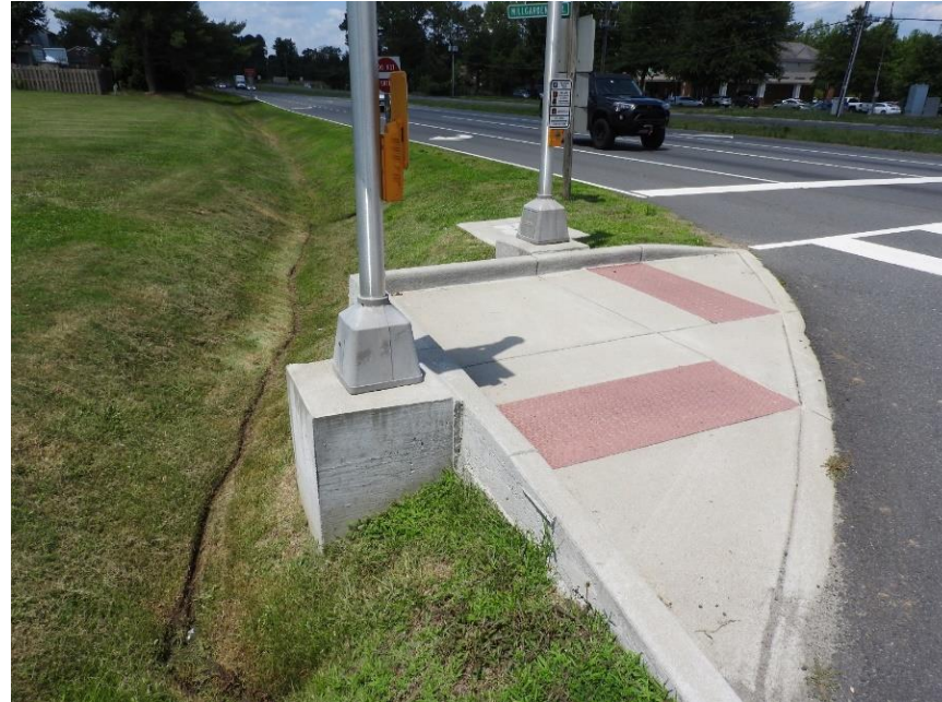
Figure 26: Example of Grade Difference at the Southwest Corner of Millgarden Dr. and Courthouse Rd. (Pictured July 2023)
