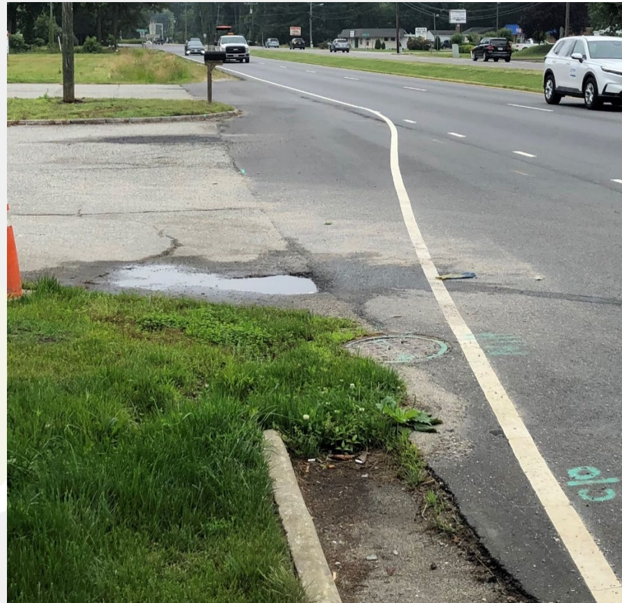
Figure 28: Photo of Lack of Deceleration Lanes and Poor Roadside Conditions
